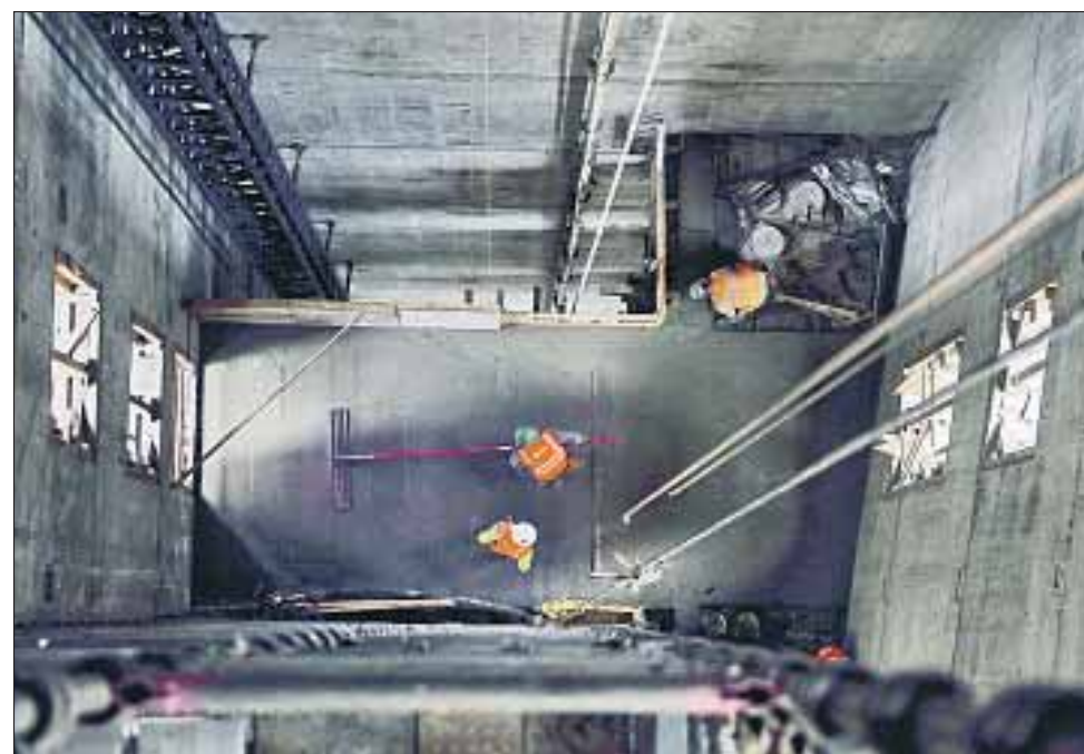
CEMENT FINISHER Jaime Velasquez, center, smooths out a concrete deck after it is poured on the 9th floor of the concrete core of the Wilshire Grand.
