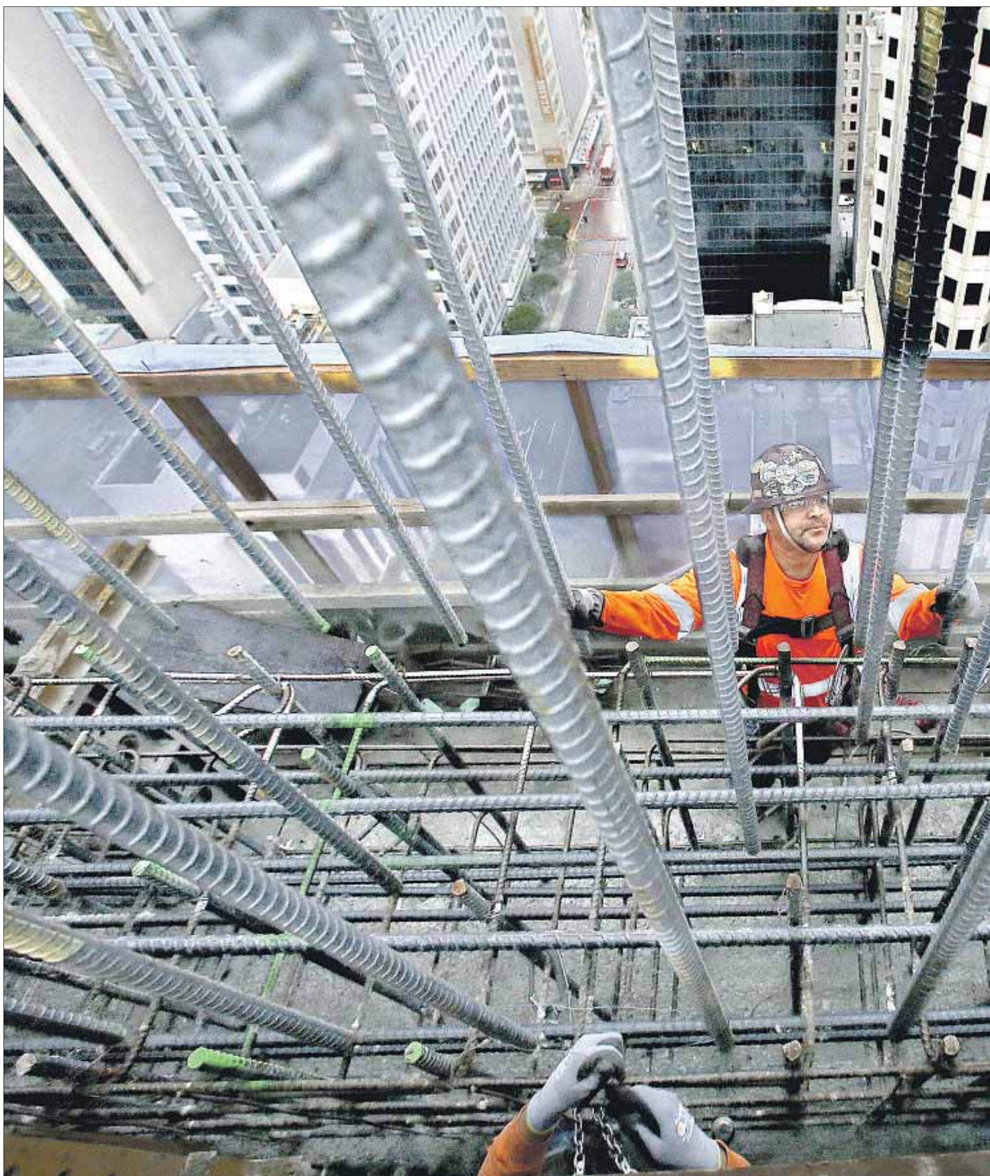
IRON WORKER Javier Jimenez guides a rebar wall into position as it hangs from a crane above. Rebar, which provides strength to concrete that would otherwise crack
