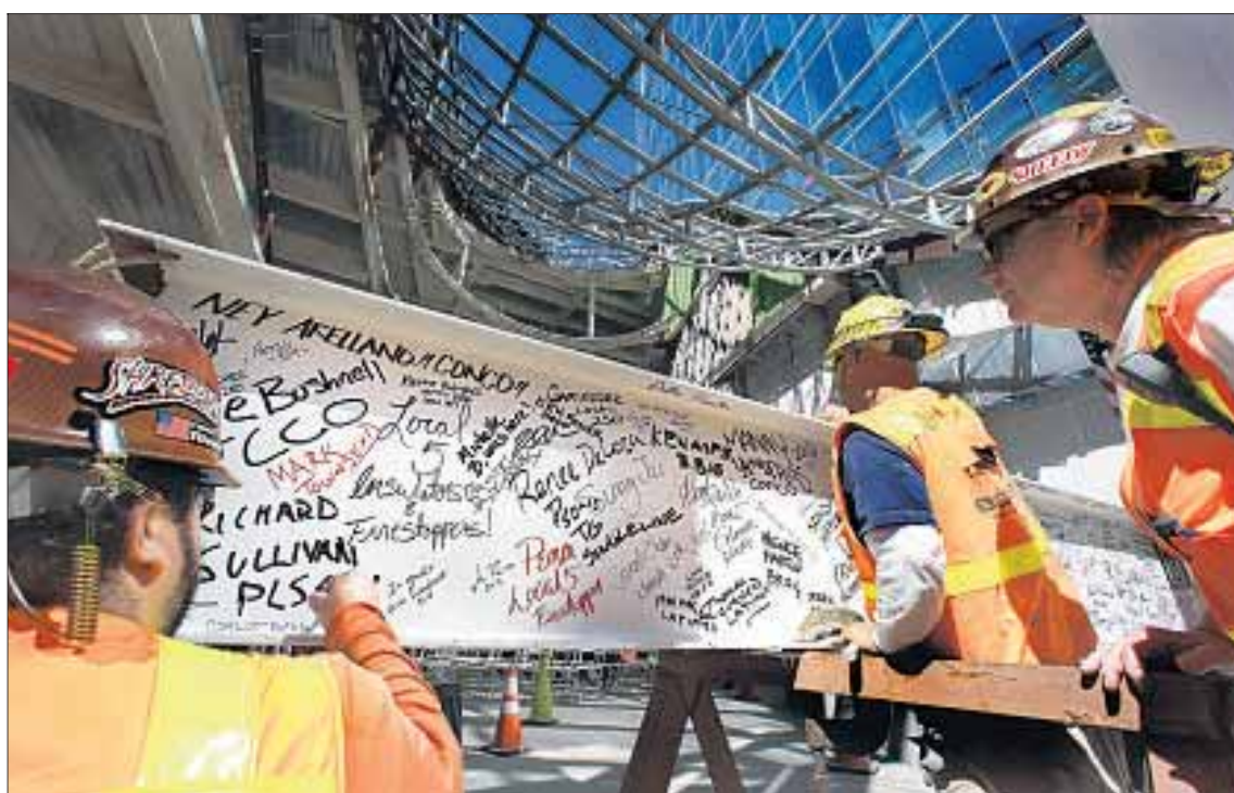
GLASS FOREMAN Gary Wahlenmaier, right, looks as glaziers Carlos Riviera, left, and Joe Guevara sign their names on a 35-foot-long, 2,100-pound steel beam bound for the 72nd floor.
