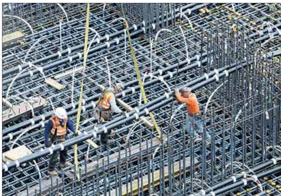
WORKERS POSITION pipes into place while standing above an 18-foot hole that will be filled with concrete to form the foundation for the project.
