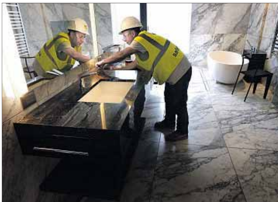
A MARBLE countertop is installed in the master bath of the Presidential Suite.
