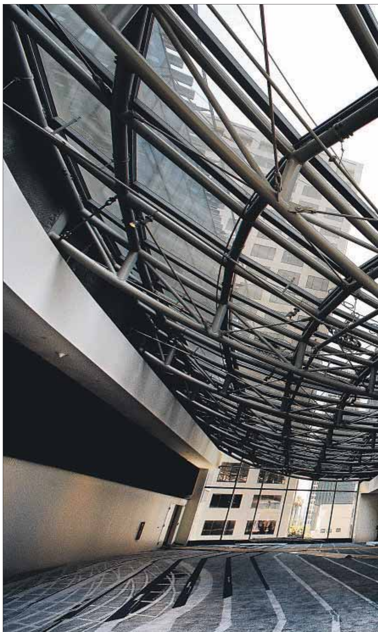
FINAL TOUCHES are made on the main path for hotel guests to get from the tower to the pool deck,
