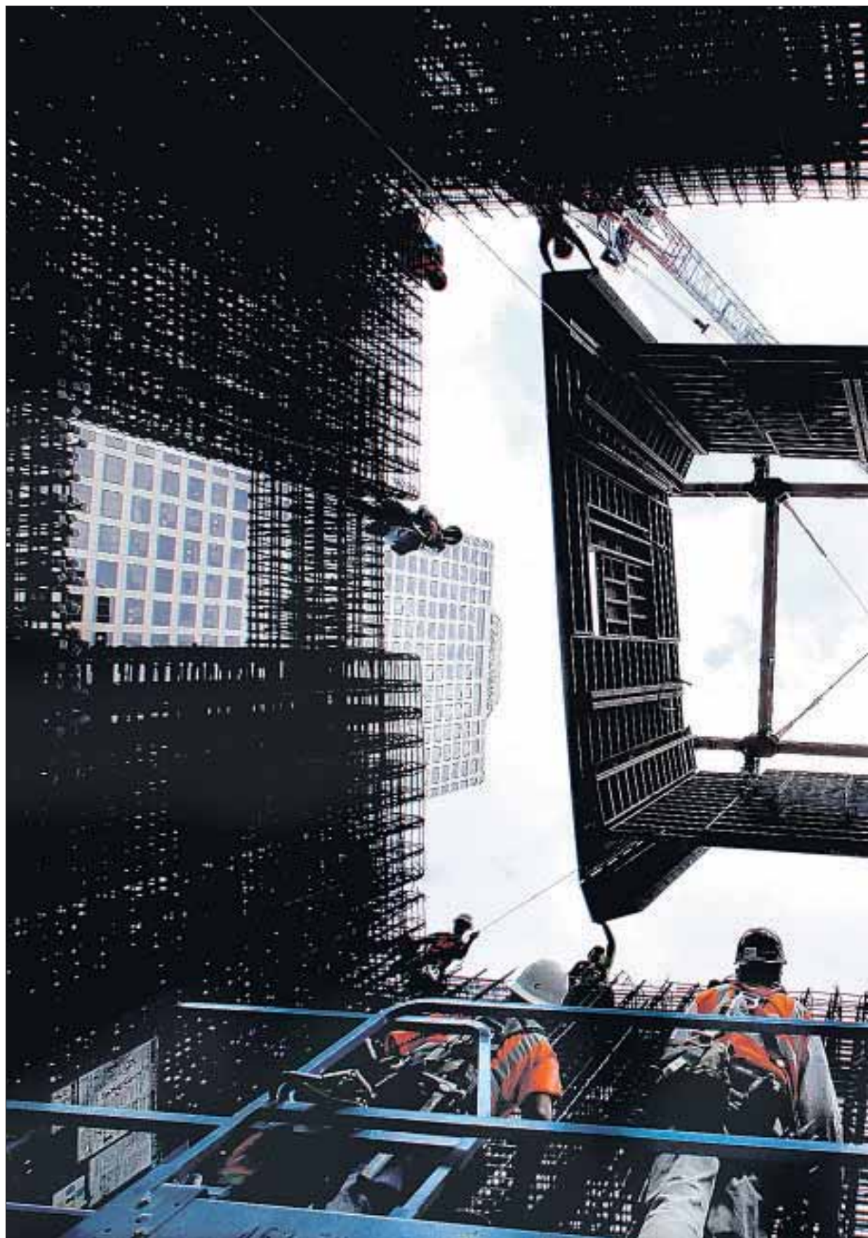
CONSTRUCTION WORKERS guide a jumping wall form system into place as it is lowered into posi-
